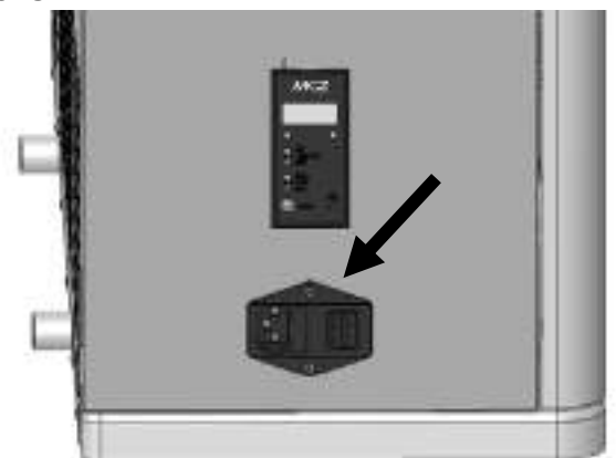
Electrical connection of the stove
