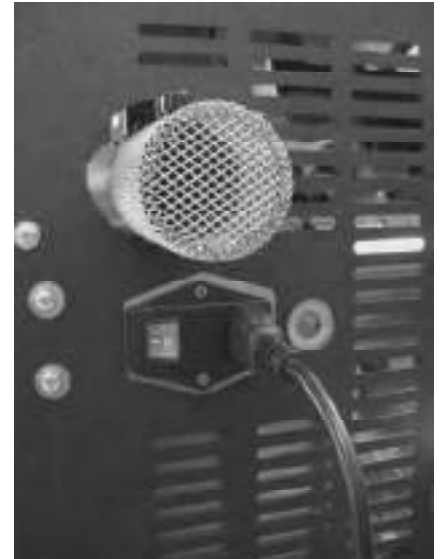
Electrical connection of the stove
